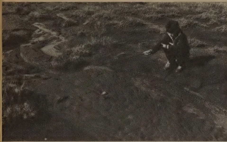
Freshly silted-in dam. Water flow is from right to left. Note the broad flattening of the streambed upstream of the sod dam. Future runoff will more easily overflow the channel and diffuse its energy over a much broader area.
